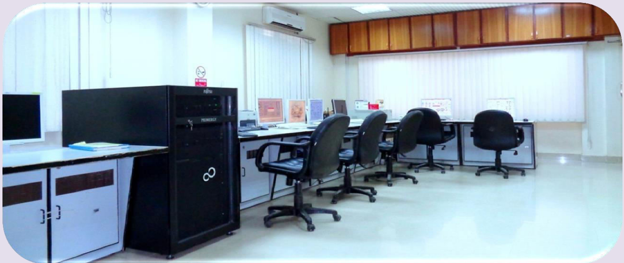
Engineering Work Station (EWS)
